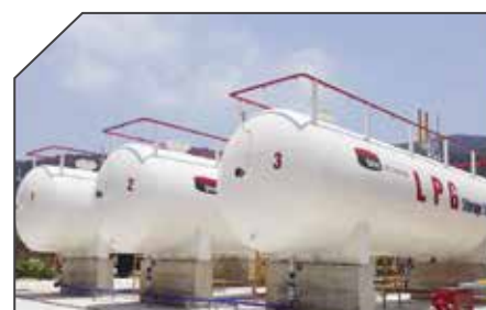
Bồn chứa LPG LPG storage tank 液化石油气储罐
